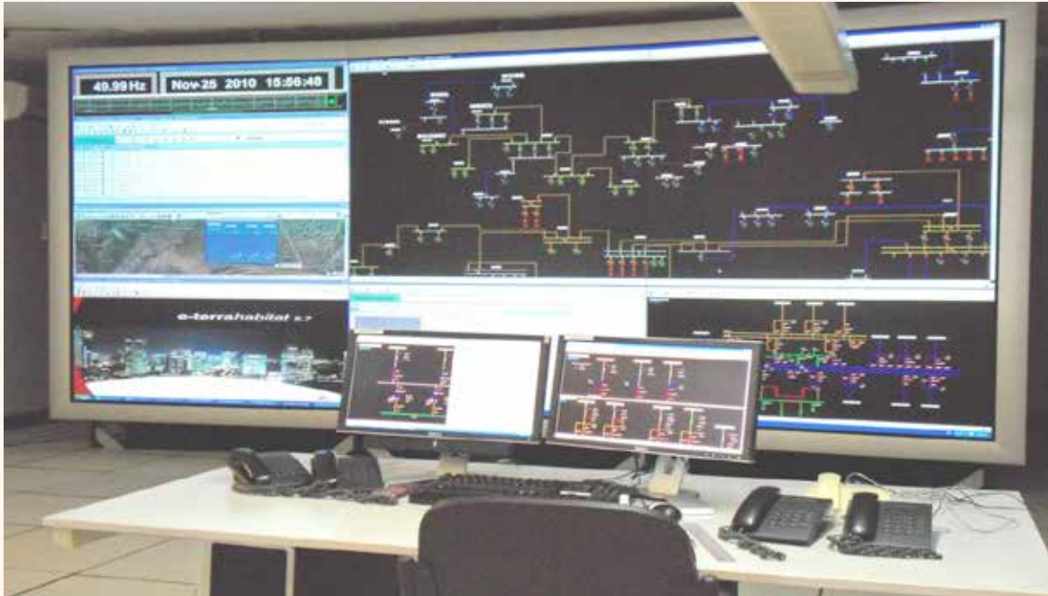
SCADA System Wall Display for Monitoring & Control of the System
