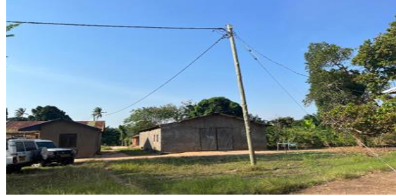
Electricity distribution infrastructure
